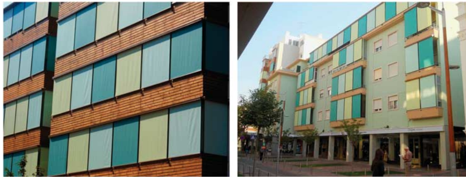
Figure 15: Av. Santos Mattos. General views of the new sunshades and matching colour scheme.
